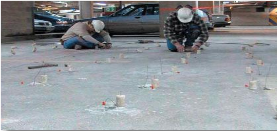
Discrete anodes for corrosion prevention in park deck
